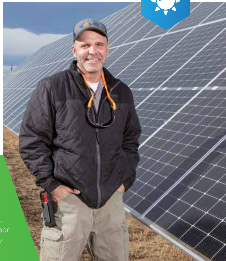
(Left) Bannon Powell, left, and Ethan Hillyer, right, with The Solar Guys, install solar panels at a job site near Cheyenne, Wyoming. Photo by Matthew Ilder Photography
